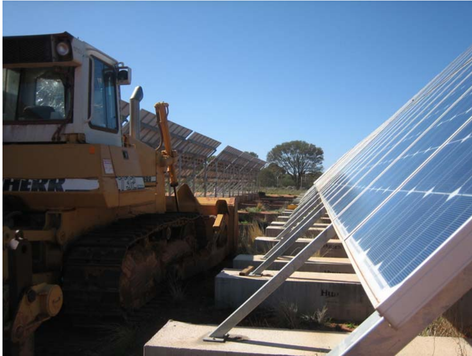
A bulldozer from Oak Valley Contracting parked amongst solar panels in Oak Valley, Officer Basin, South Australia (Great Victoria Desert).
